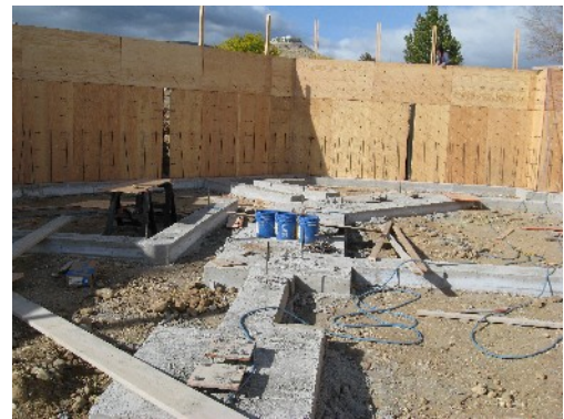
FIG 1: FOUNDATIONS Poured and STRUCTURAL BASEMENT RETAINING WALLS IN THE PROCESS OF BEING FORMED.
