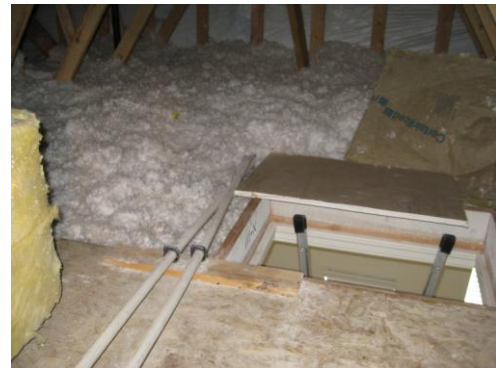
FIG 6: PLATFORM FOR THE ATTIC MECHANICAL EQUIPMENT.
