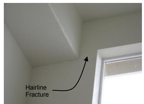
FIG 3: MINOR HAIRLINE FRACTURE AT CORNER OF STRUCTURE.
